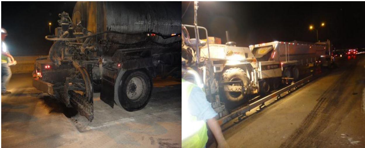
Figure 39. Existing CRCP Condition and Construction of RAP/RAS Test Sections on Loop 820, Fort Worth.
